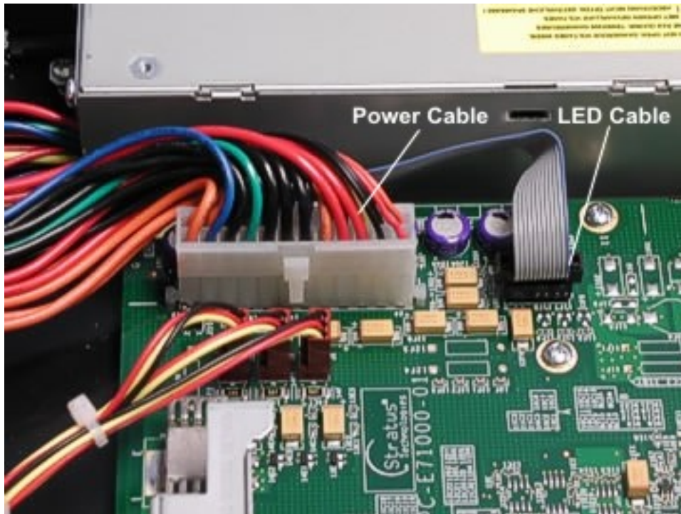
Figure 4-81. Power Cable and LED Connections at Expansion I/O Board
