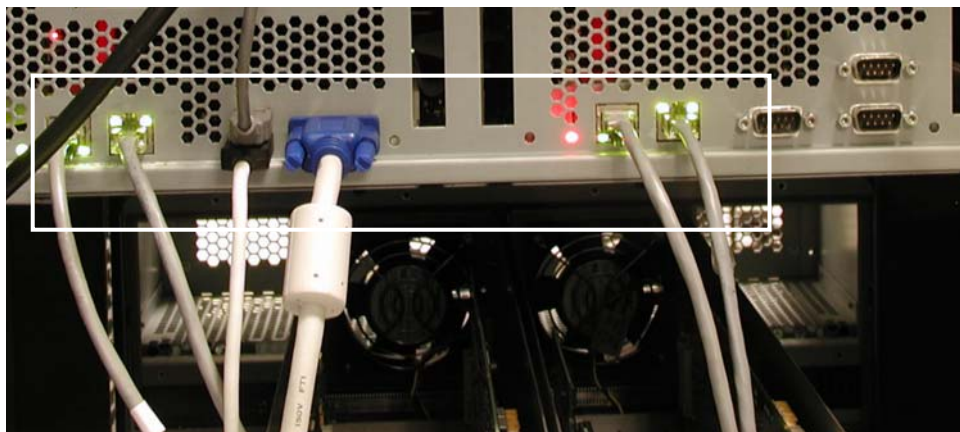
Figure 3-4. Cables at Rear of System
